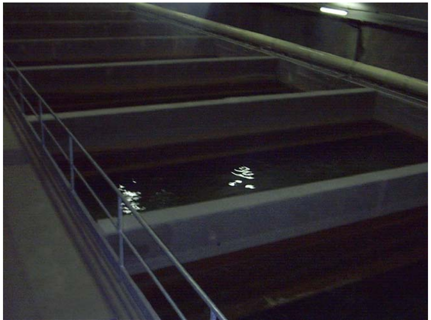
Detail about one of the basins used for the water purification system.
